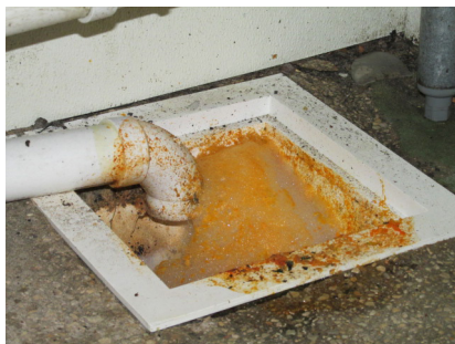
Excessive grease entering the floor drain from a dishwashing sink. Using best management practices in your kitchen can help to prevent overloading your grease trap.
