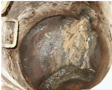
Grease flowing into the sanitary sewer from a food service establishment service line.
