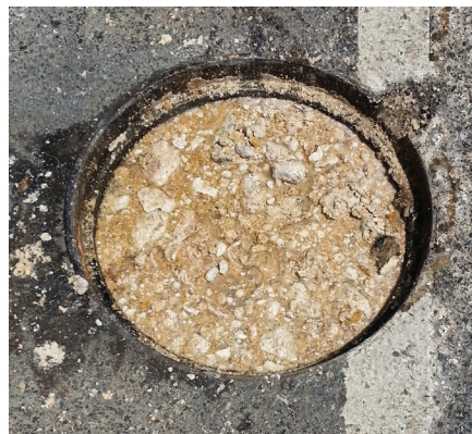
A city manhole choked by grease which passed through a poorly maintained grease trap.
