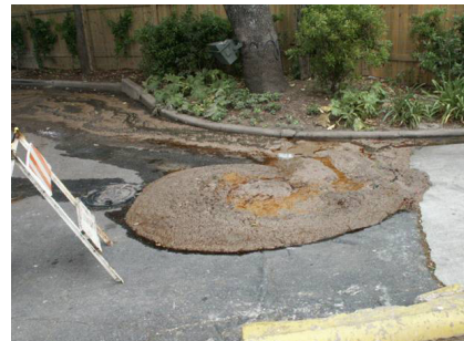
An overflow from a grease trap in the parking lot of a food service establishment.
